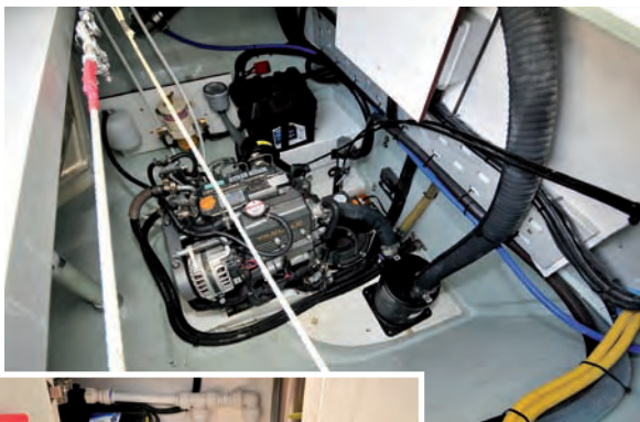
Maintenance access is ok for someone not too big. Note the filters and coolant reservoir mounted on a laminate panel rather than being screwed into the composite
