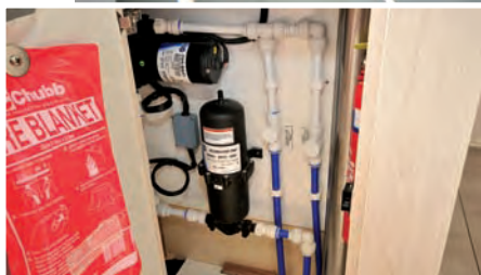
Easily understood plumbing, with fresh water pressure pumps grouped together in a galley locker. I liked the thermo-engraved labeling
