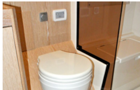
Electric toilet with sea water flush
