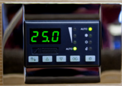
Air condition (33.000 BTU) with 4 outlets
