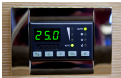
Air condition (26.000 BTU) 3 units
